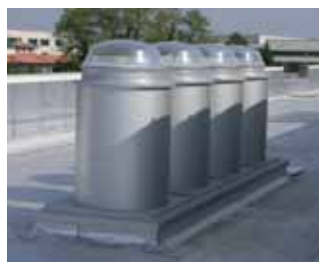
Bearing and square-based flashing with cylindrical flue and transom flashing (Massalengo school 2009)
